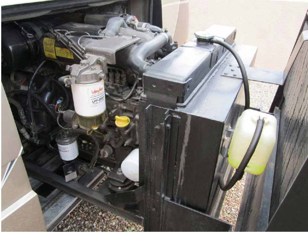
20KW Turbocharged Diesel Generator
