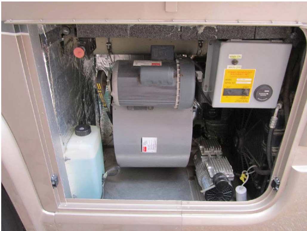
Generator blower and 12V air compressor
